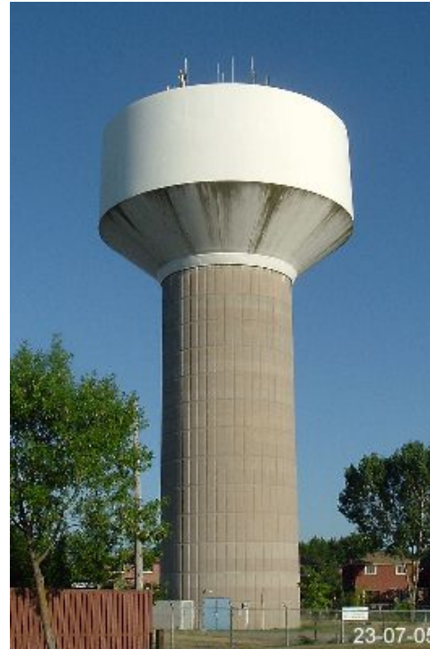
York Region elevated tank with visible dark staining on conical section.
