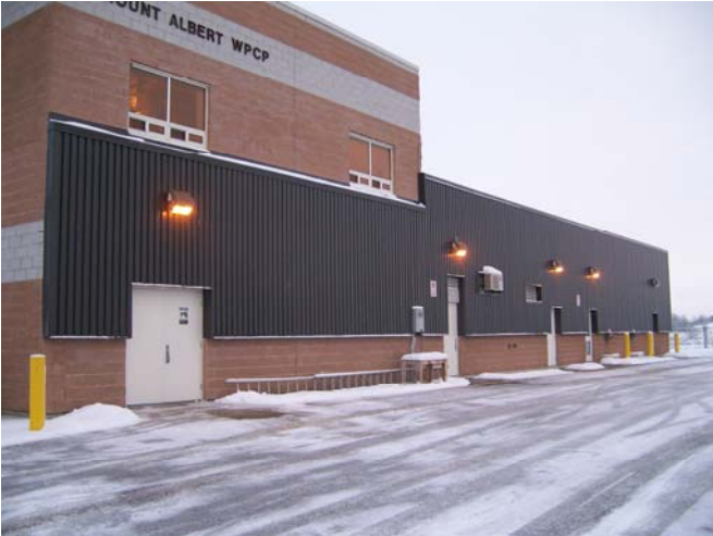
York Region's first SolarWall® air heater installed at the Mount Albert Water Pollution Control Plant.
