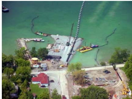
Georgina Water Treatment Plant – Lake Simcoe Intake
