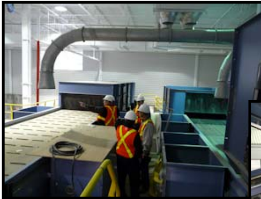
Temporary Picking Station
