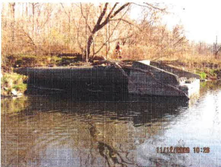
Figure 1. The effects of lateral migration on a typical storm sewer outfall.
