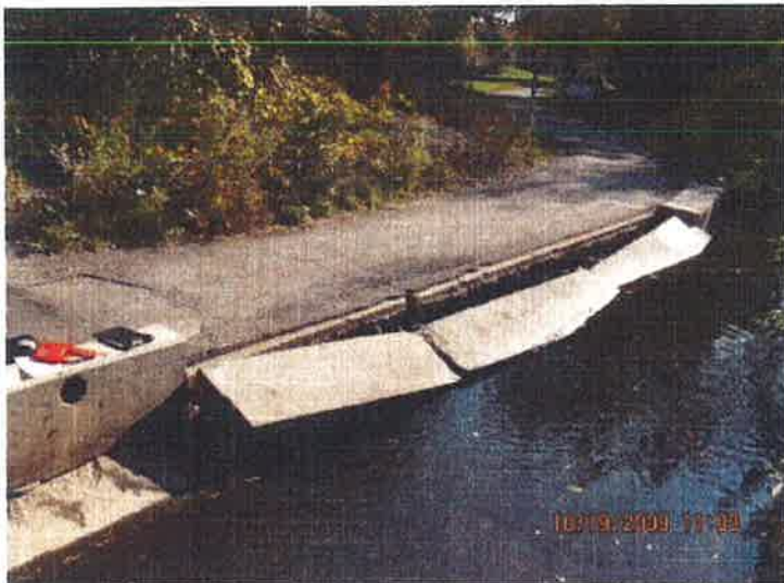
Figure 2. Failures like the one above appear to have overnight and are often not budgeted for, but must be addressed quickly to protect public safety
